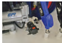
DC DEF Pump
