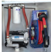
Inside Front Box with 25 GPM, 12V DC Pump
