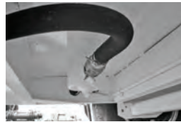
Fuel Shut Off Valve
